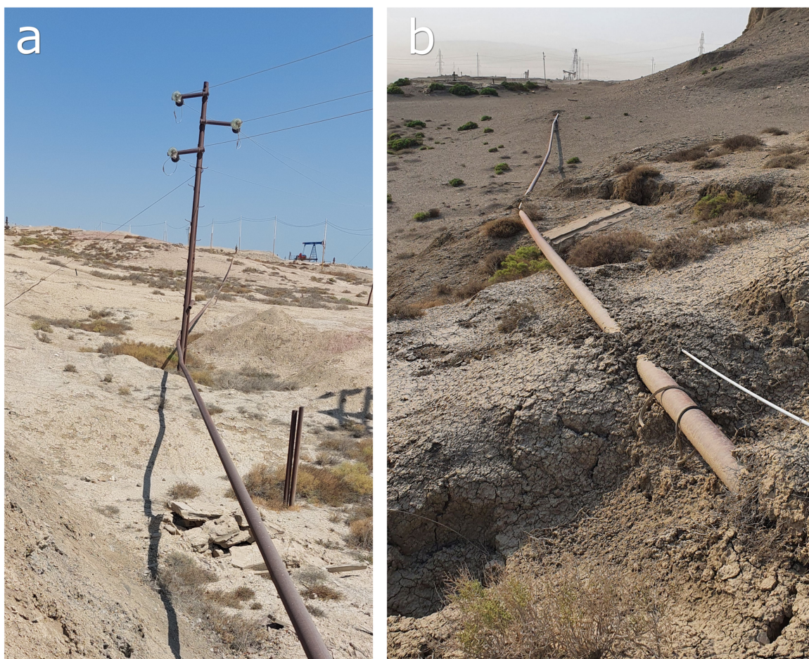
Figure 5: Example of infrastructures built across the creeping mud flow at Lokbatan MV. (a-b) ongoing flow movement causes deformation of the pipeline.
